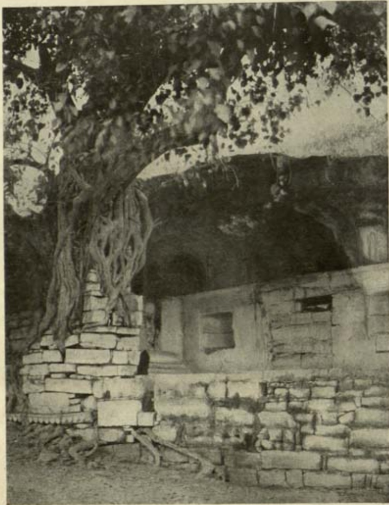
Old palace, Sassaram, District Shāhābād, Bihar: ficus on structure with roots penetrating and striking ground
