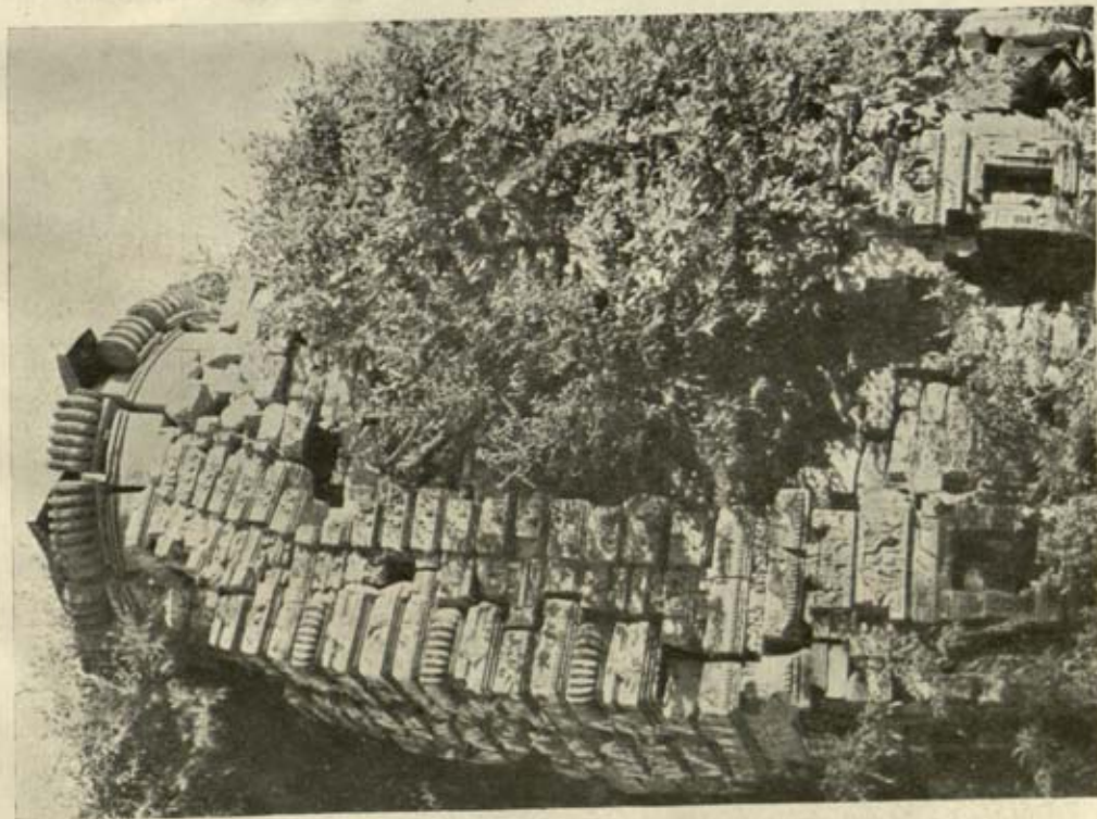
A. Ruined temple near Kojitīrthā, Bhuvanesvar, District Puri, Orissa: woody shrub on vimāna bursting out the structure
