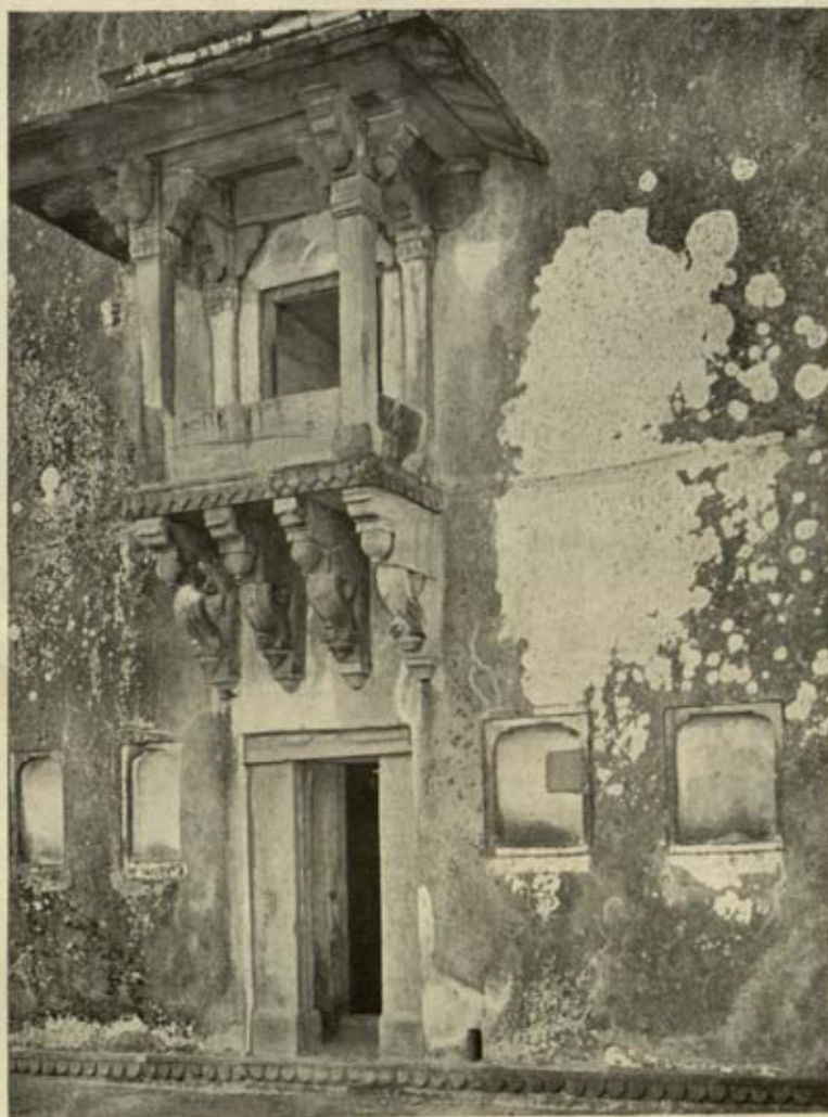
Rohtas fort, District Shāhābād, Bihar: large patch of lichen on the right of the balcony and sporadic patches on the left
