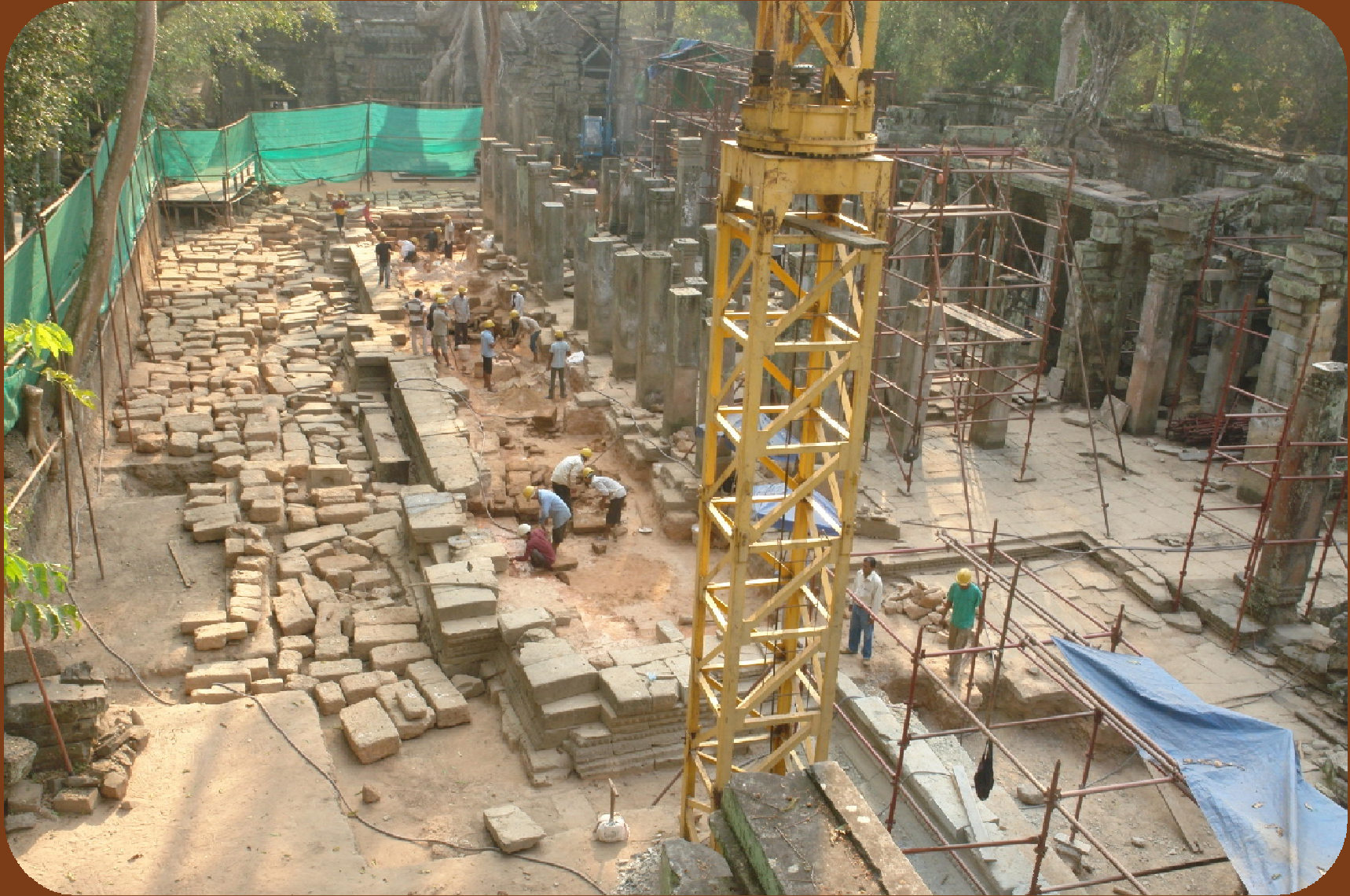
Hall of Dancers - Inter northern floor after removal of sandstones and laterite stones.
