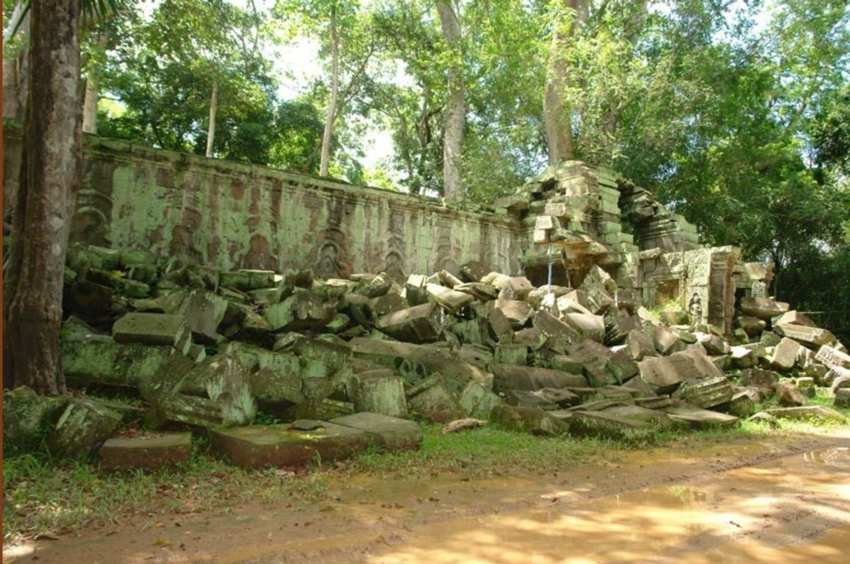
Collapsed third Enclosures Gallery on North East , Ta- Prohm, Temple Archaeological Survey of India
